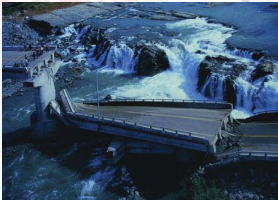
Figure 1.1 : Damages caused by 6m displacements reverse fault in 1999 Chi-Chi Taiwan (after Stanton, 2013)
