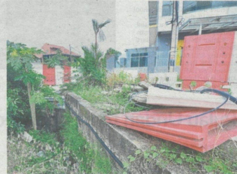
Construction hoarding and material too close to existing premises along Jalan Raya Satu in Serdang Jaya
