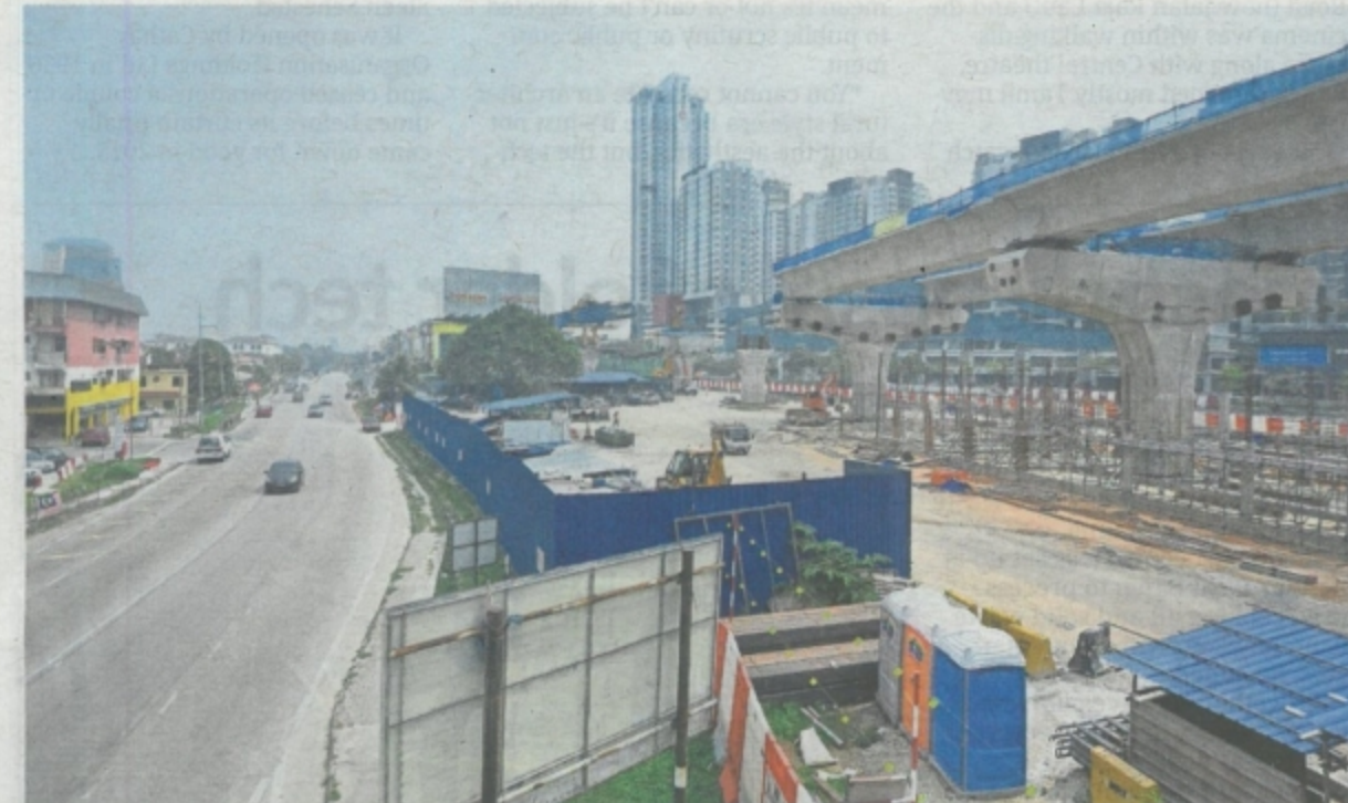
Also known as MRT2, the SSP Line is progressing ahead of schedule.
