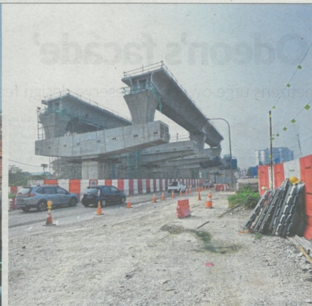
With roads in Seri Kembangan and Serdang Jaya already narrow, it is not easy for the massive MRT2 construction sites to be located at a distance from the road, away from motorists and buildings.
