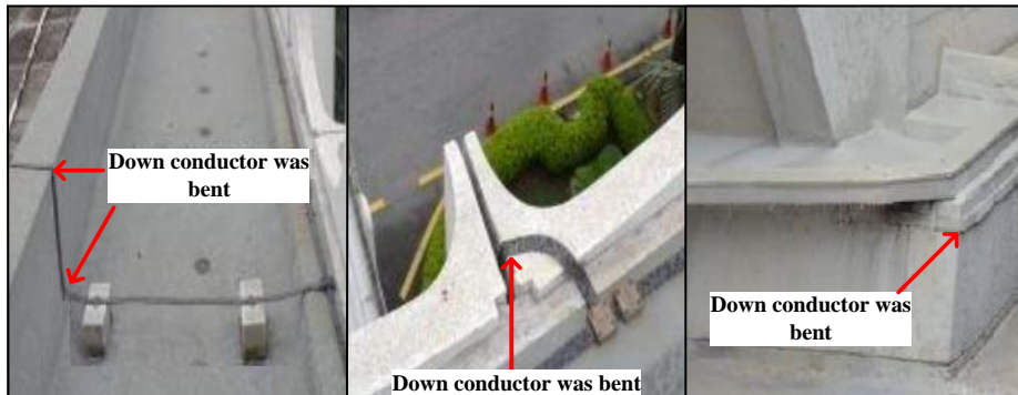
Figure 1.1: The practical installation of down conductor is bent due to the structure of the building [10]
