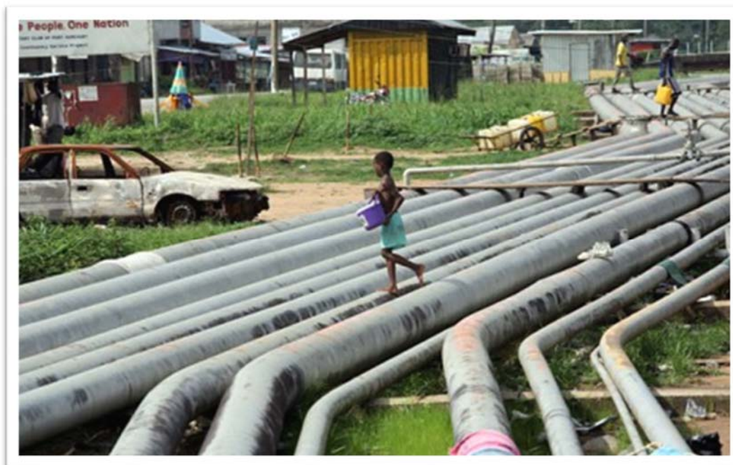
Figure 1.5 : Pipelines crossing through Village. (Source: AI (2009))
