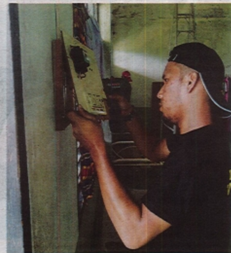
A Politeknik Mersing student earning extra income doing electrical wiring, a skill related to his field of study.
