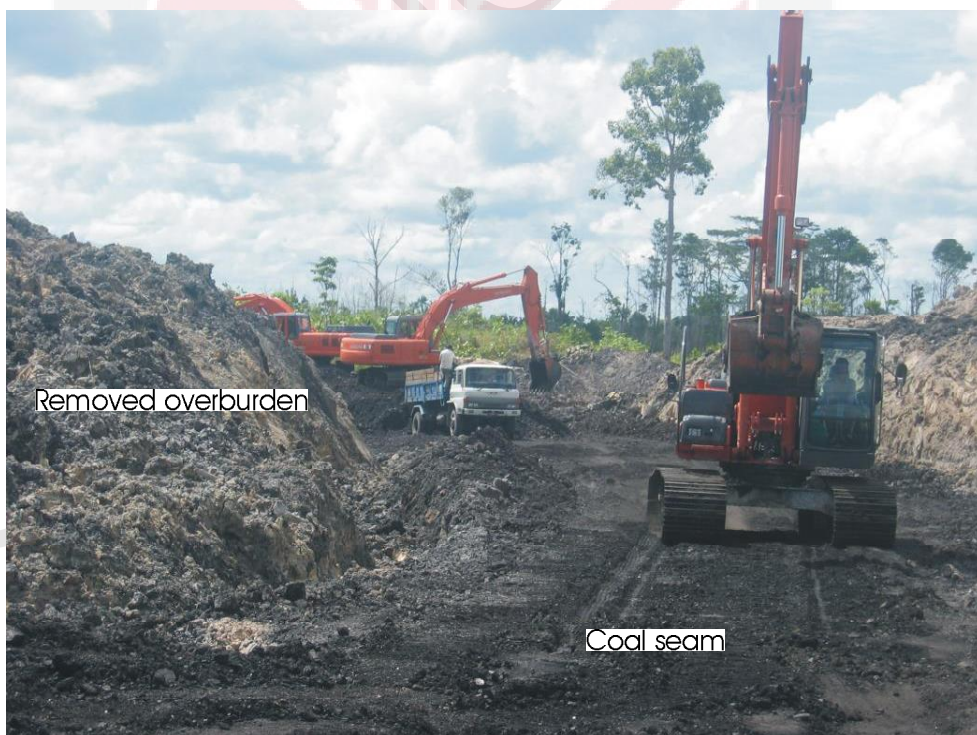
Figure 1.2. Excavating coal and transport it to stock pile at Kampung Jebungan Mukah
