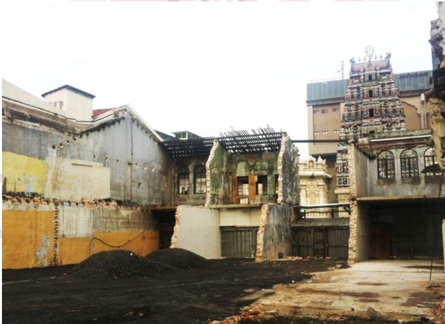
Figure 1.5 – Kuala Lumpur Chinatown Few Heritage Shophouses were Demolished With Façades Retained. One of them was Total Lost.
