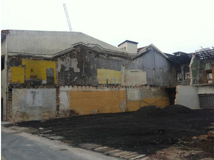
Figure 1.9 – Demolished of 4 Units of Old Shophouses at Jalan Tun H.S. Lee. Old Shophouses User Demolished the Entire Building for New Development. Image source: Y.S. Toong
