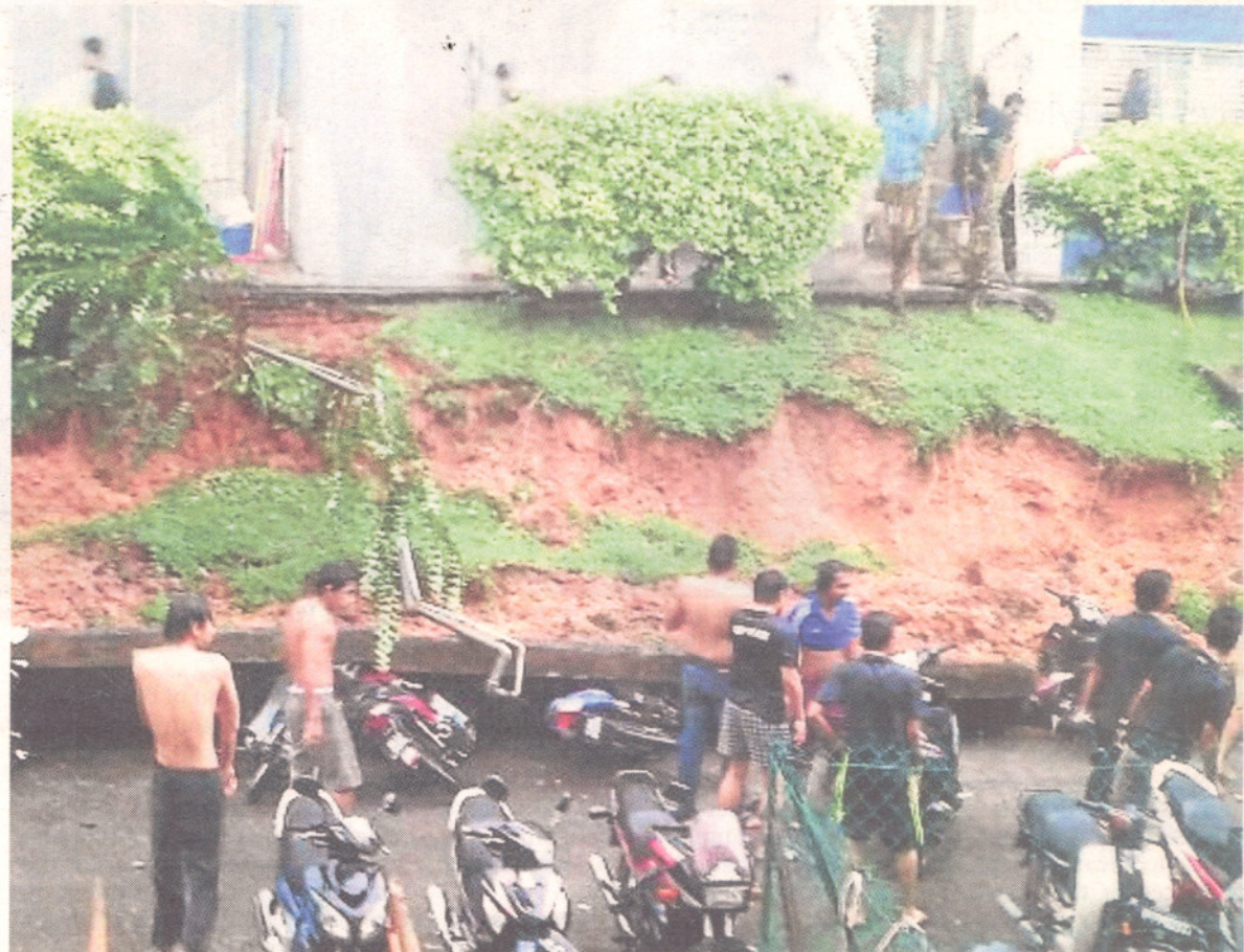
Universiti Putra Malaysia students surveying the damage caused by the landslide at the parking area of their college. Pic by Asyraf Sawal
