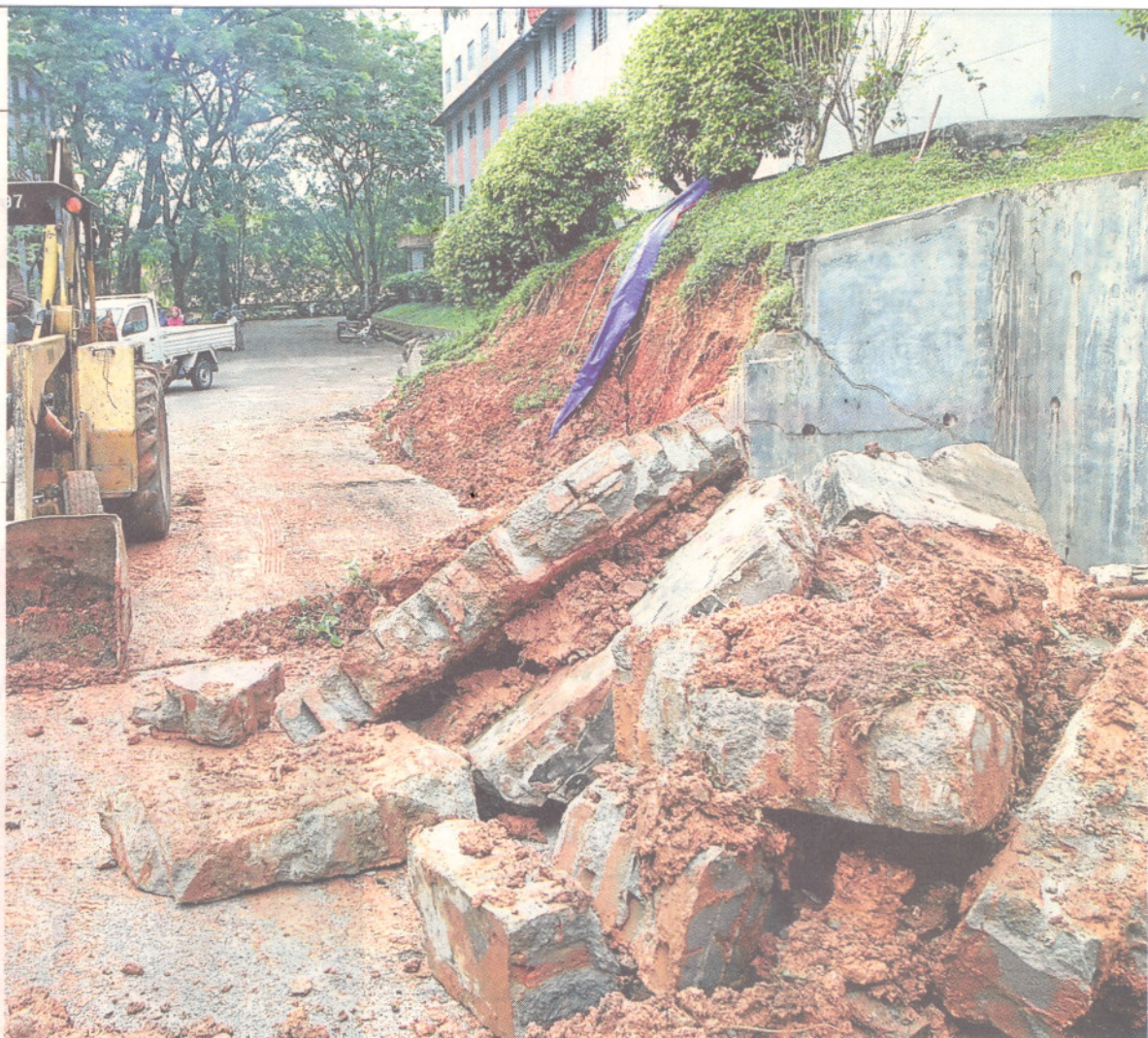
A portion of the damaged retaining wall yesterday, which collapsed at a residential college in Universiti Putra Malaysia in Serdang on Friday. Pic by Mokhsin Abidin
