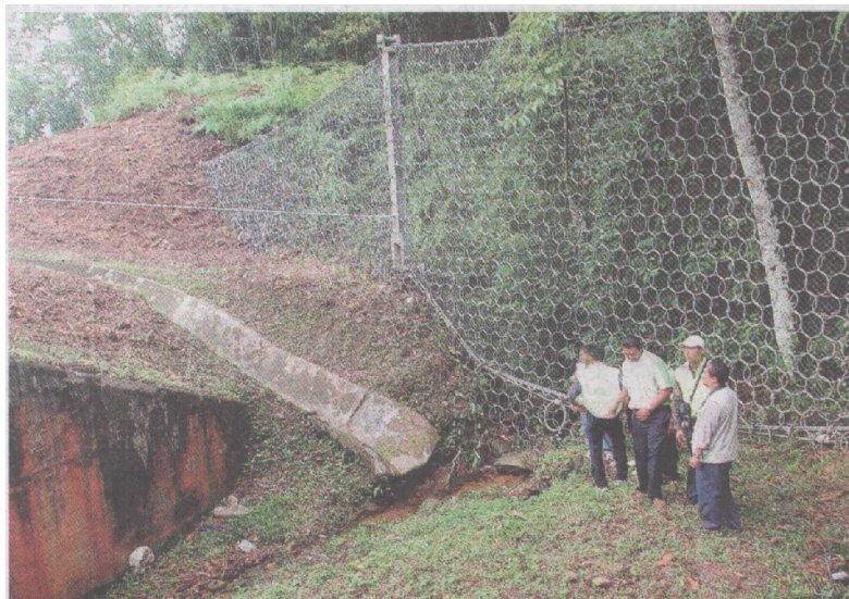
One of the five debris flow nets installed at Gua Tempurung and Jelapang.
