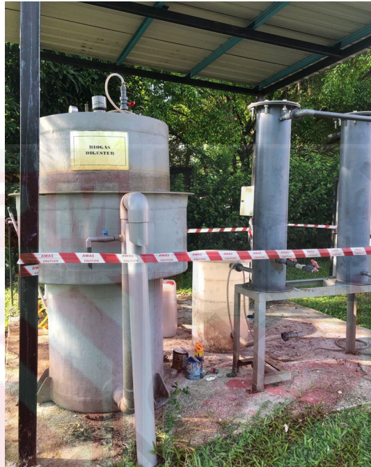
Figure 4.18: Setup of 500 L AD system at food premises for the project purpose.
