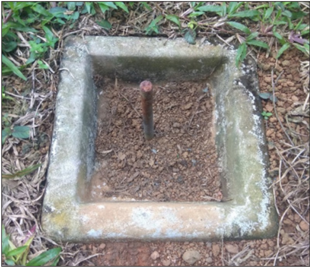
Figure 5. One of the untreated earthing electrodes (EE-3)
