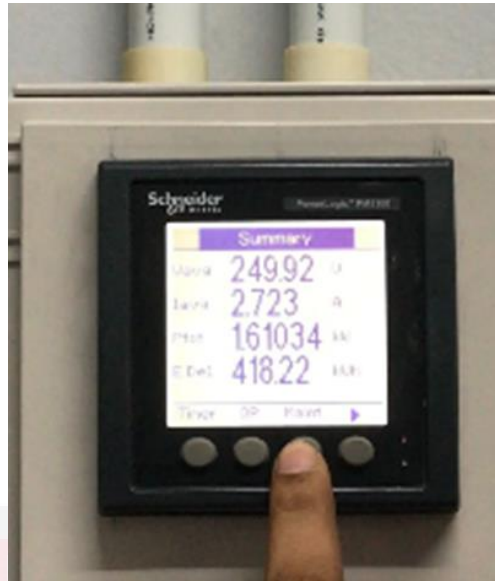
Figure 4.4: Reading shown from power meter sensor, Schneider PM5110.
