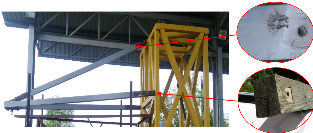
Figure 2.4: Lightning and environmental degradation issues on cross-arm lead to structural damage. (Source: Rawi et al. (2017))
