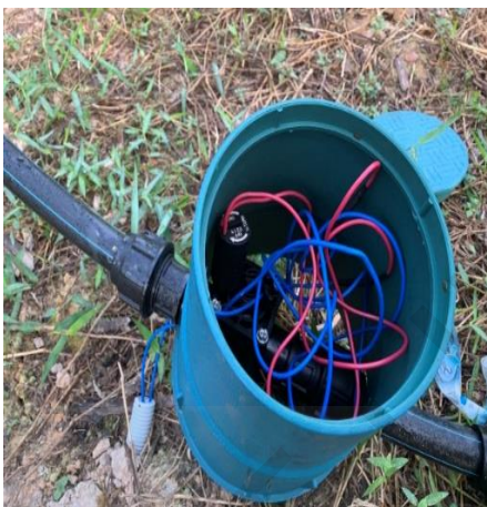
Figure D.21: Solenoid valve installed at sub main pipe
