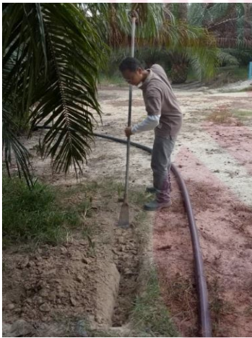
Figure D.5: Some part of the main pipe was buried in the soil for safety purposes
