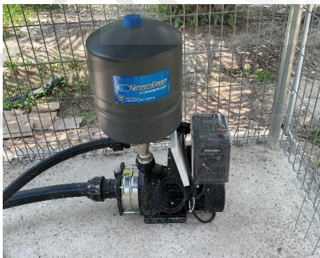
Figure D.7: Electrical pump unit to draw water from the tank
