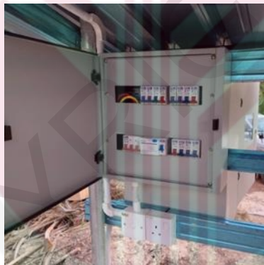
Figure 3.30: An electrical control board was installed near the water tank
