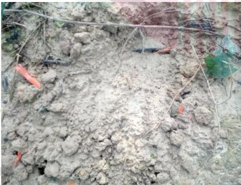
Figure 4.53: Lightning strike affected wire buried in the soil
