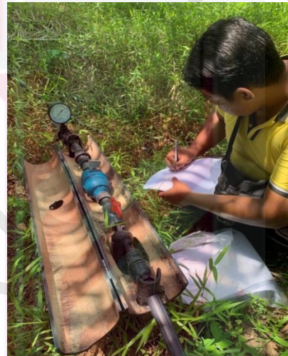
Figure D.6: Several parts for monitoring purposes were installed on this segmentation
