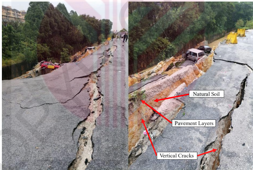
Figure 3.18: Landslide failure showing cracks condition since 2001 showing the soil type in the construction area not changed
