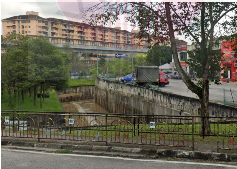
Figure 3.16: The area before landslide failure (Date of picture January 2021)
