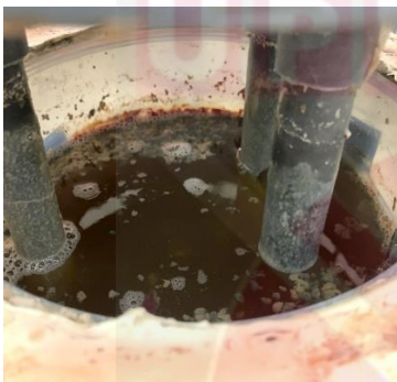
Figure 4.10: Sludge residues on the surface of Tank 1
