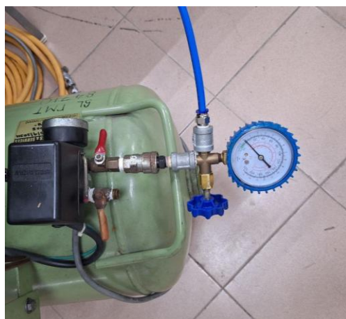
Fig. 4. Pressure gauge of the air compressor to control inlet pressure
