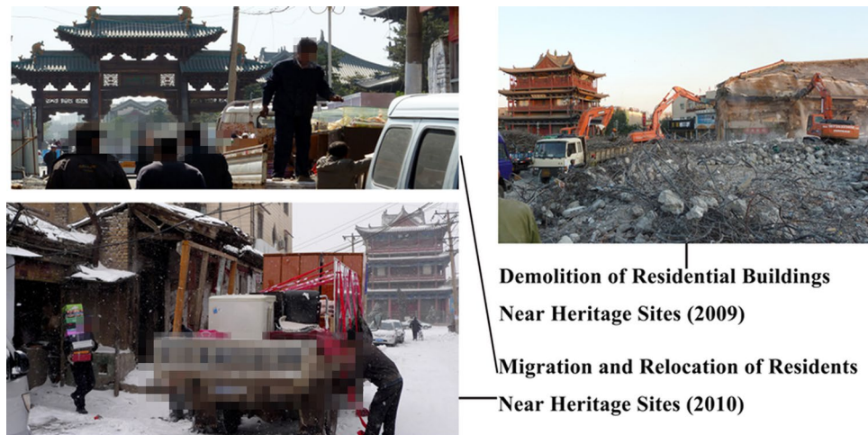
Figure 5. Reconstruction of Datong Ancient City: Demolition of residential buildings near the ruins and the large-scale relocation of residents.
