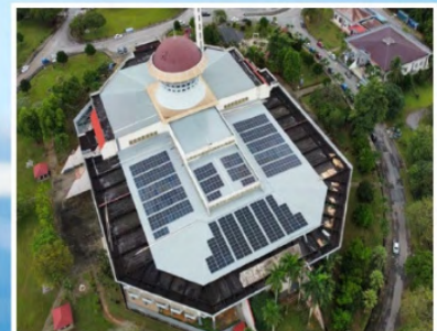
Masjid UPM (415.80 kWp)
