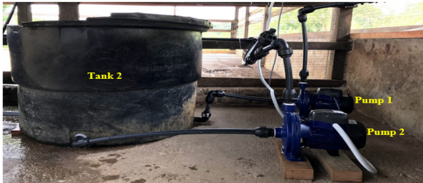
Figure 3. The water-conducting network from Tank 2, two centrifugal pumps and filters
