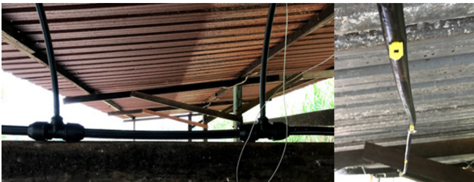
Figure 4. Distance between water ducts, which were smaller diameter than water channels (left), and the placement of misting spray nozzles along the water ducts (right)
