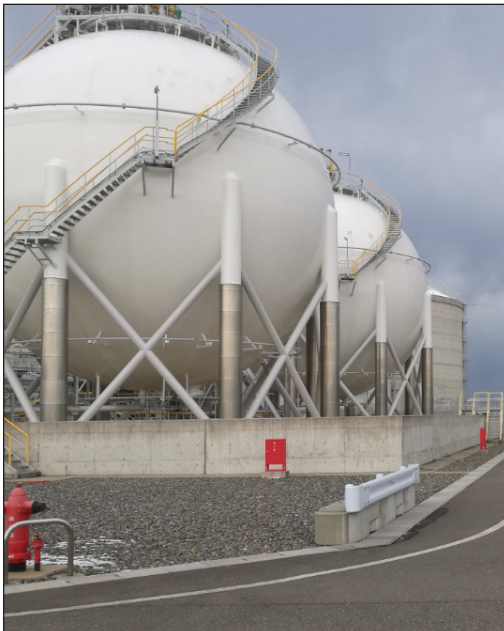
Figure 6. INPEX LNG regasification terminal - bund around LPG sphere
