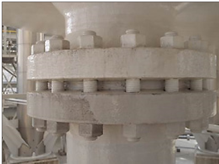
Figure 4. INPEX LNG regasification terminal - Non-leak flange
