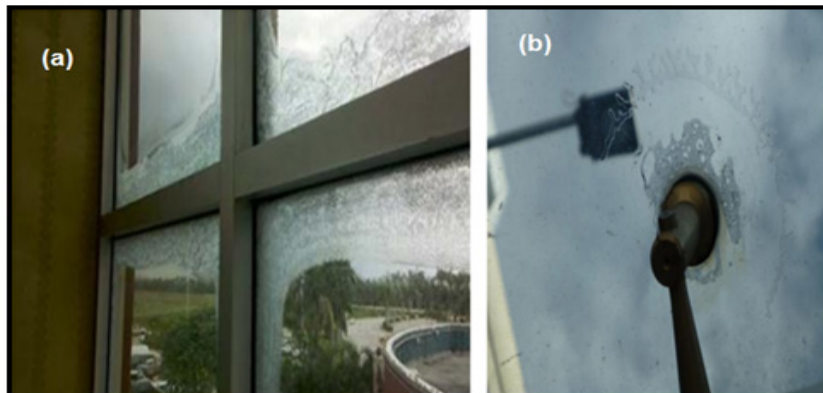
Figure 2. Delamination of LG panels (a) framed window glass (b) Point fixed glass (CPNI EBP 04/13, 2013)
