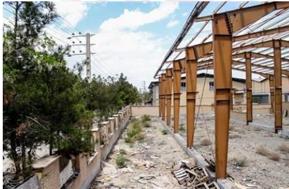
Figure 1.10 : Uncompleted industrial sheds in companies
