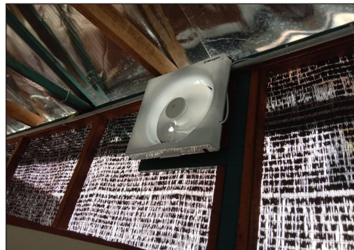
Figure 16. Ventilation fan to cool down the temperature and for air circulation
