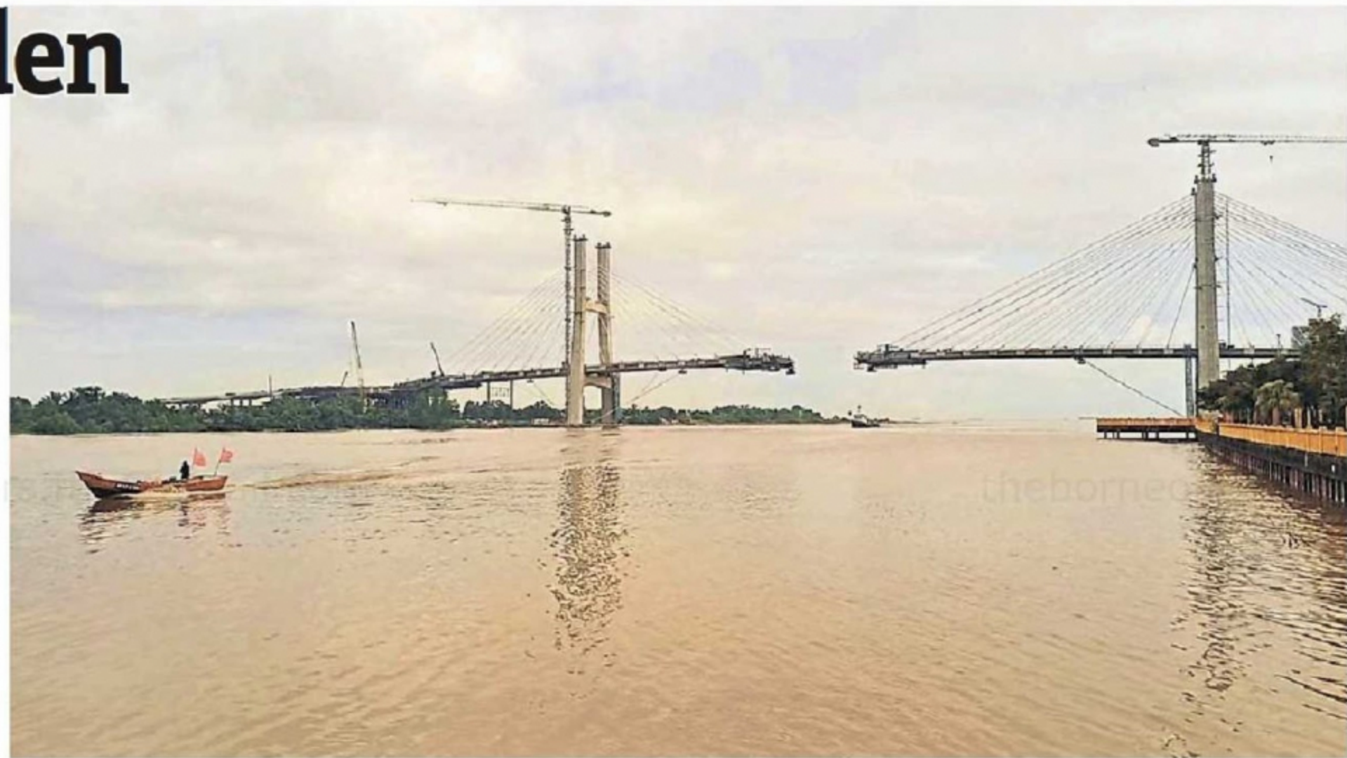
Photo of the Bintulu-Jepak bridge, which is slated for completion this year end, taken from Bintulu Waterfront Promenade.
