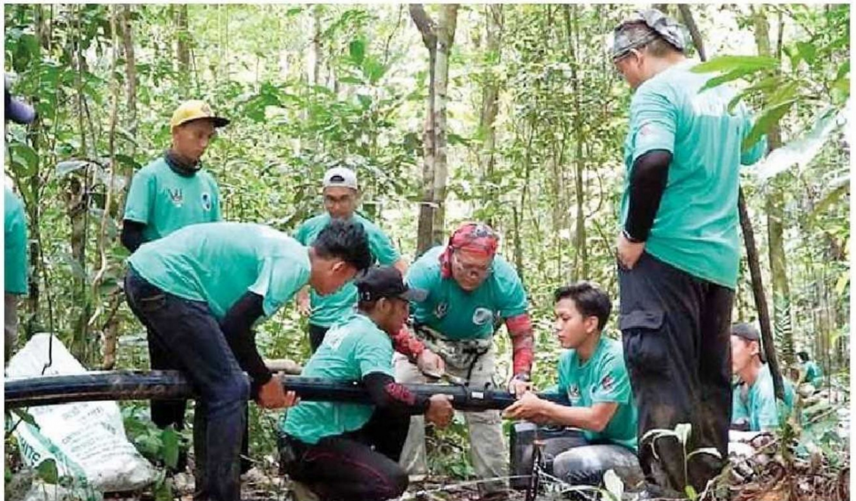
Volunteers get hands-on experience in installing water pipelines for the community project. — Photo via Facebook/UPMKB
