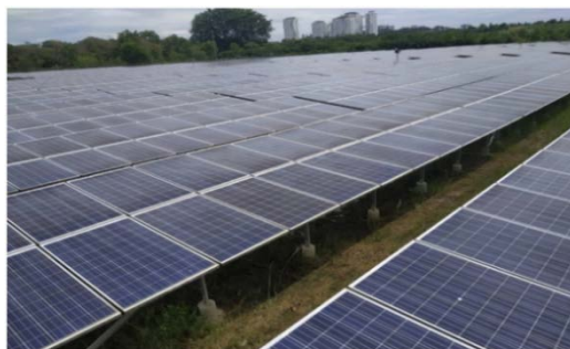
Fig. 2. 2MWp Solar Farm in Puchong, Selangor.
