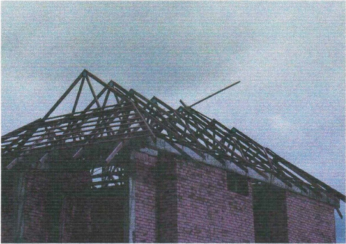
Plate 2 : Roof structure constructed using prefabricated timber roof truss for a typical double storey house
