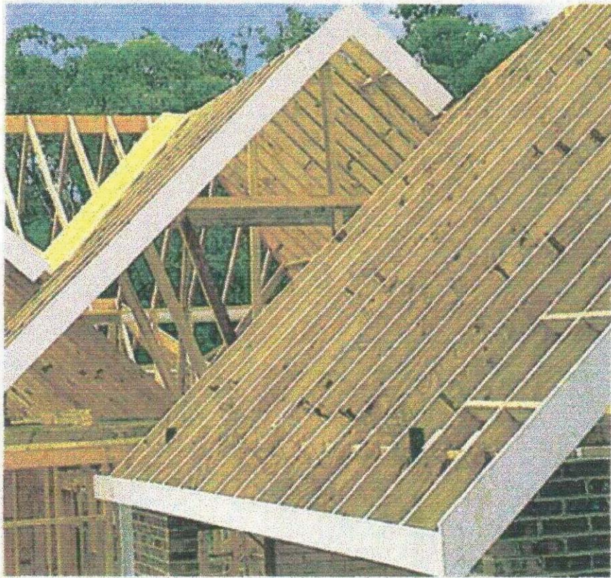
.Plate 4 : Hyspan used in construction of roof structure for residential house. (Photo taken from Hyspan © Span Tables for Residential Building. Carter Holt Harvey Wood Products, Australia. November 1997)
